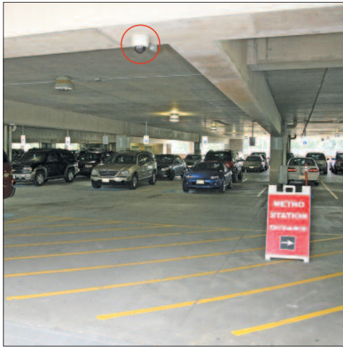
A Panasonic camera is watching as vehicles enter the Metro Centre garage. A total of 102 cameras keep watch throughout the facility.
