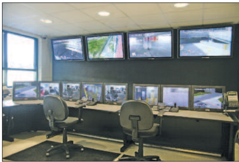
The control room features four 42-inch Panasonic plasma display monitors and eight Panasonic 20-inch LCD monitors.
