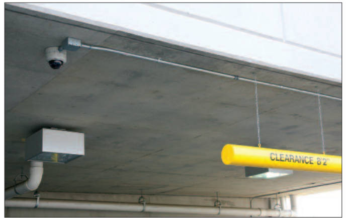
Dome cameras from Panasonic keep watch over commuters' vehicles at a nine-level mass transit parking garage in Owings Mills, Md.
