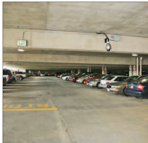
Panasonic's WV-CW964 pan-tilt-zoom dome cameras are strategically located to cover the largest possible area inside the Metro Centre parking garage in Owings Mills, MD.
