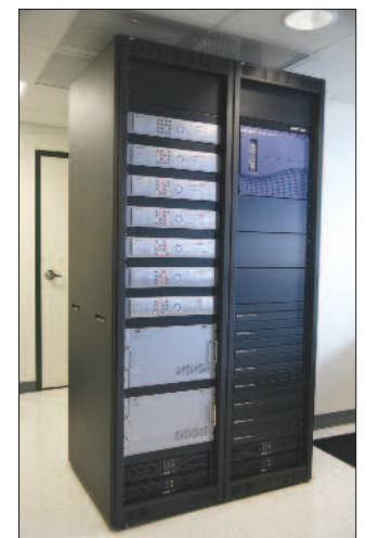
Two racks in the control room hold the Panasonic DVRs and matrix switcher, a Talk-a-Phone PBX system, the Vigitron passive hubs, an uninterruptible power supply and extended battery backup.
